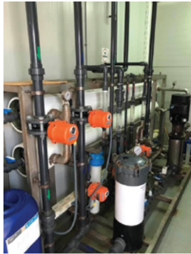
Reverse osmosis desalination unit at EJUST campus, providing safe and free drinking water
