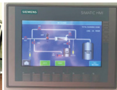
Automatic control and monitoring of the RO system
