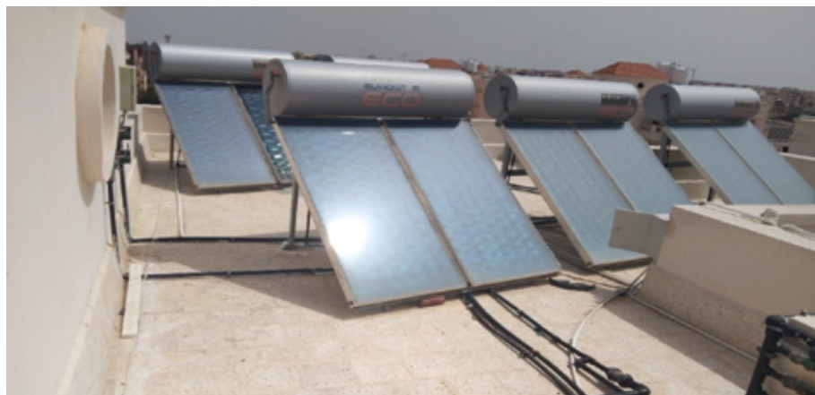
Solar water heating in housing buildings
