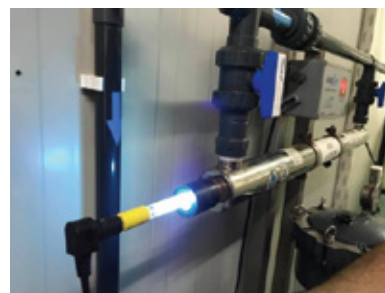
Ultraviolet (UV) unit for disinfection
